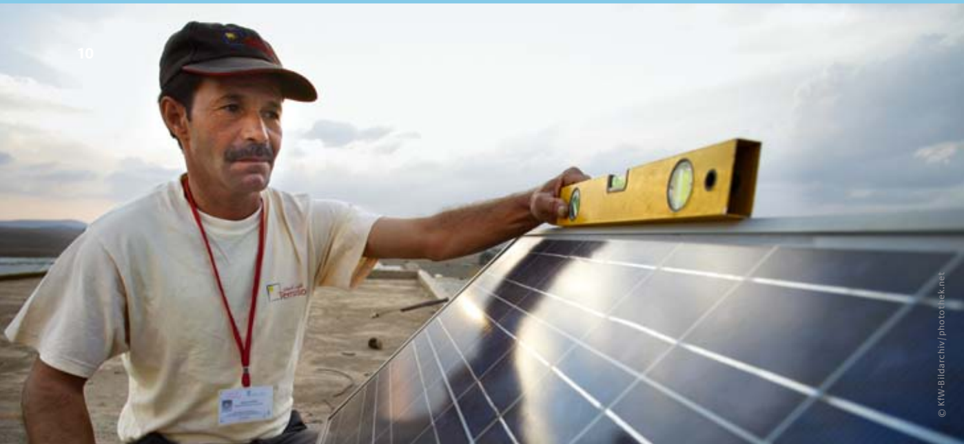
Solar power plants generate sustainable energy in Morocco.
