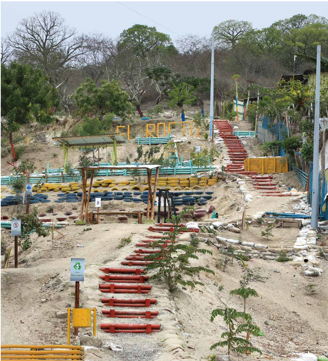
Slope stabilisations like this one in San Pablo reduce the risk of landslides even during heavy rain.
